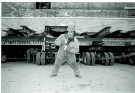
A SERIES OF DOLLIES supporting the Shubert Theater allows Rick Swaggert to move the structure down a Minneapolis street.
