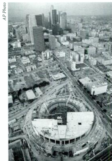
THE UNDER-CONSTRUCTION Staples Center in downtown Los Angeles is well on its way to its scheduled October completion date. The $360 million arena's first announced booking is next year's Democratic National Convention. The Staples Center, seen in this March 5th aerial shot, will be home to the Los Angeles Kings hockey team and the Lakers and Clippers basketball teams.
