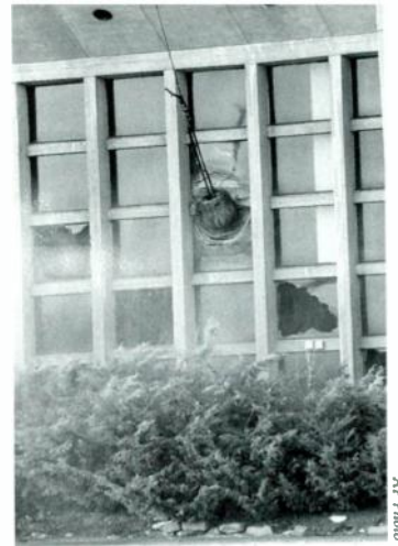
A 6,000-POUND wrecking ball smashes into the side of the Richfield Coliseum in Ohio. Demolition of the 20,000-seat venue on the edge of Cleveland began March 30th. The former home of the Cleveland Cavaliers was sold to the National Parks Service and will become part of the Cuyahoga National Recreation Area. The building has been dark since the NBA team moved to the Gund Arena in 1994.
