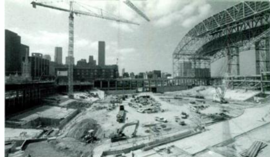
THE RETRACTABLE-ROOFED Enron Field inches its way toward completion in time for next year's opening day. The Houston Astros will move to the new ballpark next season. Enron Energy Services unveiled the stadium's name April 7th and will pay the team $100 million over 30 years for naming rights.
