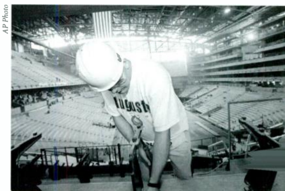
A CONSTRUCTION WORKER bolts in support brackets for the seats at the Philips Arena in Atlanta. The $213 million venue, set to open in September, will seat up to 21,000 for concerts.
