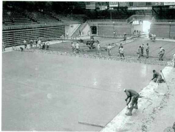
SOUTH DAKOTA'S Sioux Falls Arena recently completed a $1.7 million renovation, which includes a new ice hockey floor. The venue's renovation began in May and was completed July 31st.
