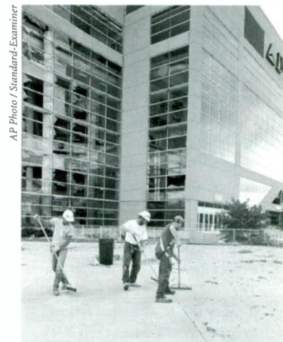
WORKERS SWEEP UP GLASS in front of the Delta Center August 11th after the tornado that shocked Salt Lake City.
