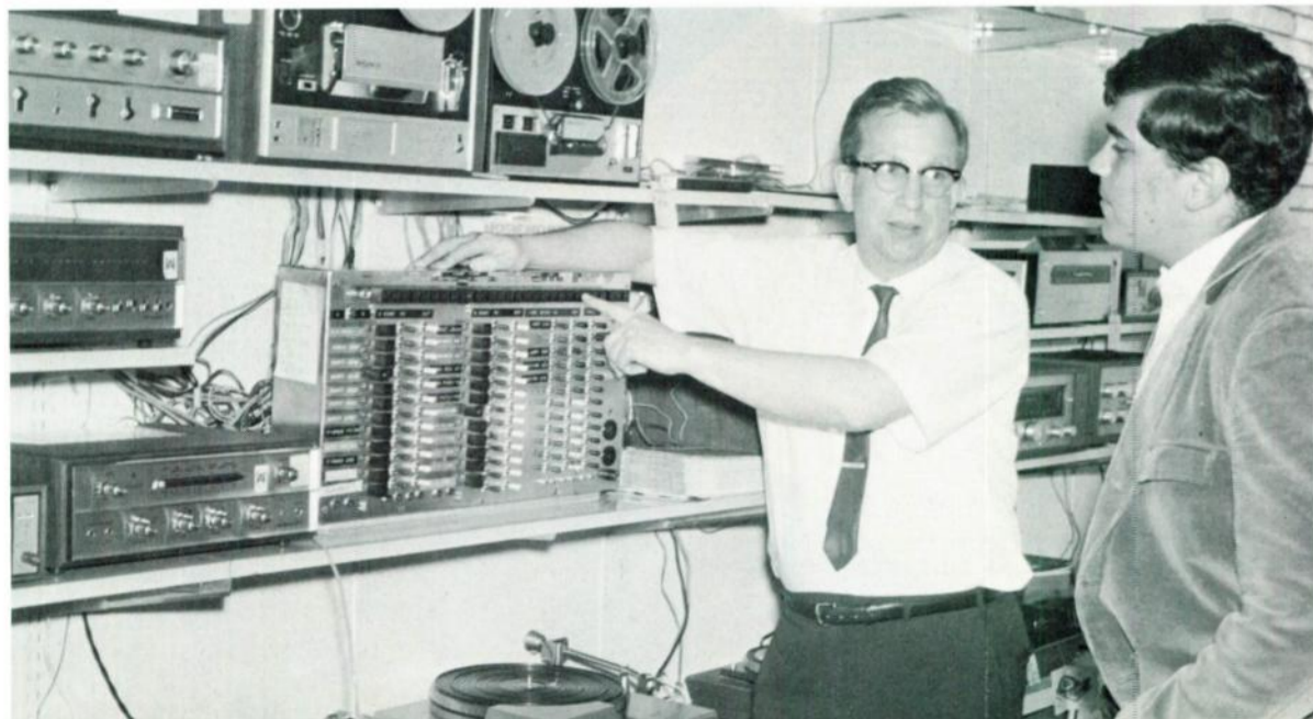
Control panel for switching combinations of music systems and speakers is shown to prospect by F. T. Beecher.
