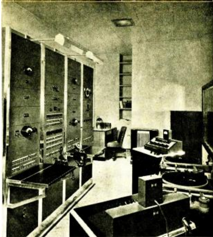
Speech input equipment at Station WOW, Omaha, Nebraska. (Photo courtesy Western Electric Co.)
