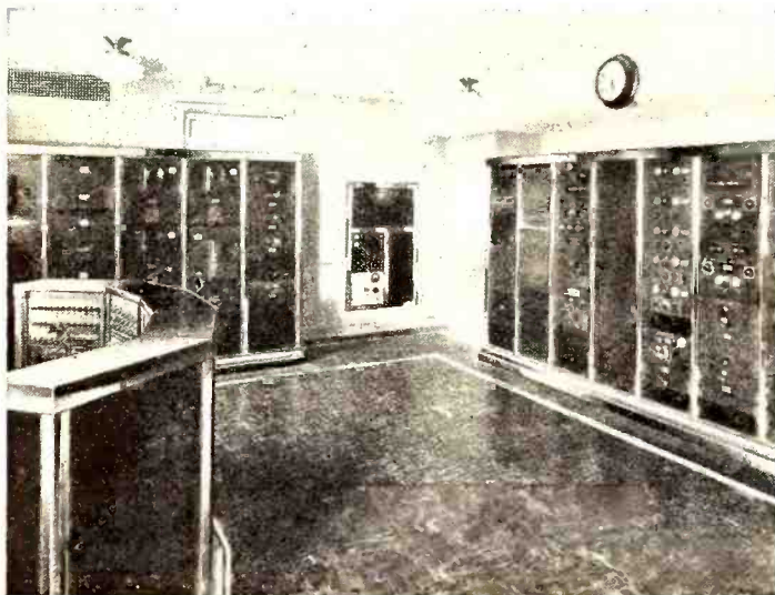
Rectifier Panels are at the Left and Audition and Line Amplifiers at Right in this General View of WHK's Master Control Room. The Chief Operator's Desk is in the foreground.
