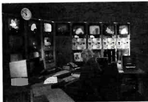
Rational Automation System installed at the Pennsylvania Public Television Network, Hershey, PA.
