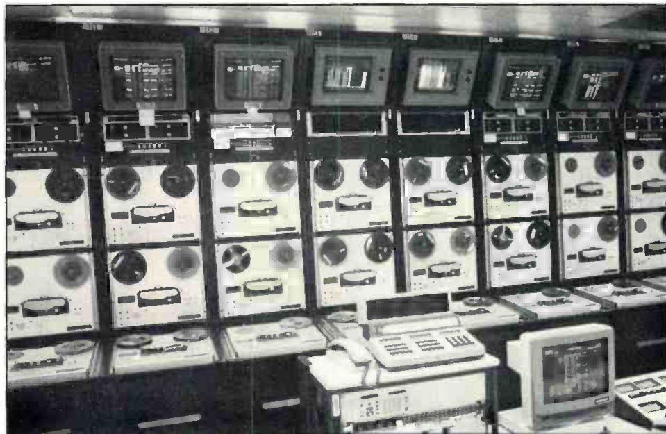
New master control room at RFE/RL's headquarters in Munich. Each rack represents the feed to a transmitting station. Up to 16 feeds can be sent simultaneously.
