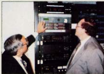
Dr. John King, director of wvxu(FM) Cincinnati, and Gerald LeBow, president of Sage Alerting Systems, flank the first installed Sage ENDEC system.
