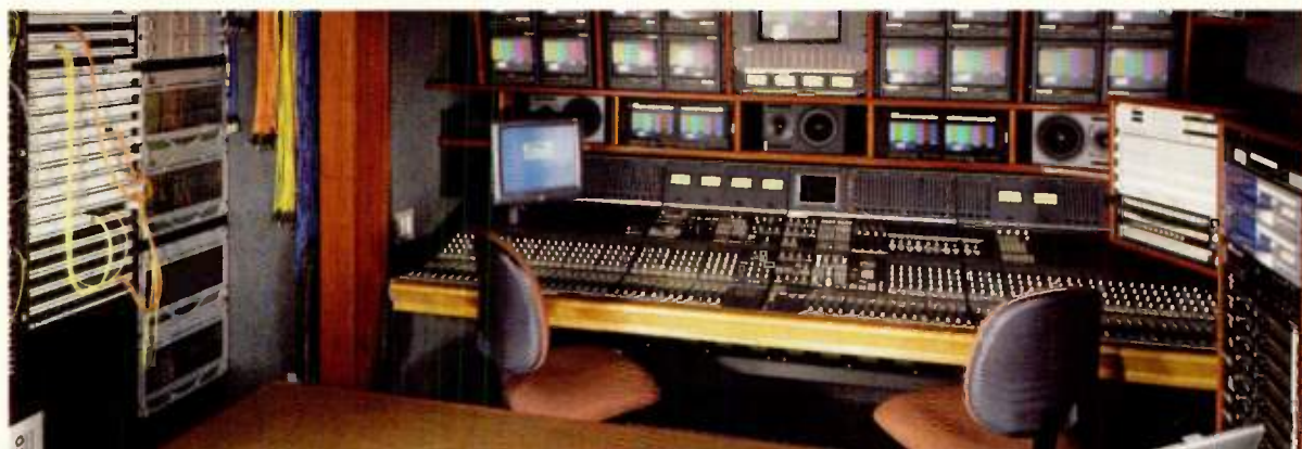
The SS24 has the largest control room of any production truck.
