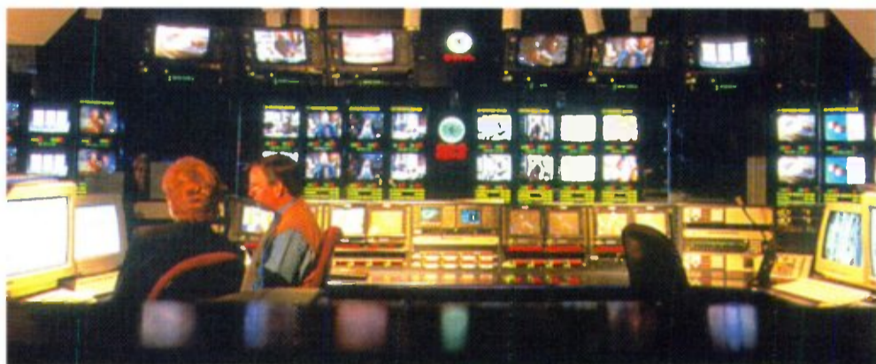
NBC is transmitting its HDTV feed from a facility in its Rockefeller Center-based Genesis plant.
