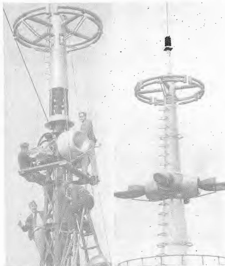
NEW TELEVISION antenna being built for operation by RCA-NBC atop the Empire State Bldg., New York. Left photo shows antenna being erected for test at the RCA Communications laboratories at Rocky Point, Long Island. Right photo shows how it will appear when installed.
