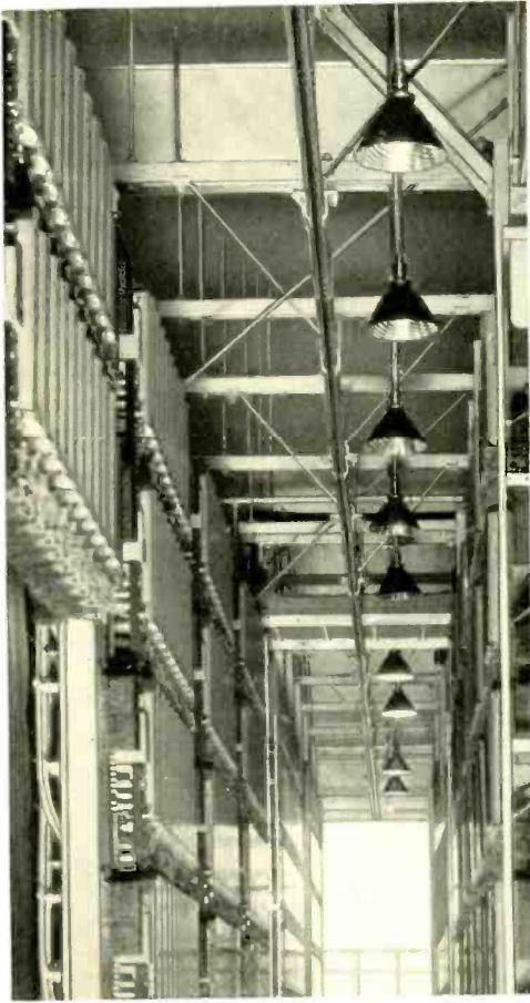
Fig. 2—In switch rooms mirrored glass reflectors are commonly employed to give the higher intensities required
