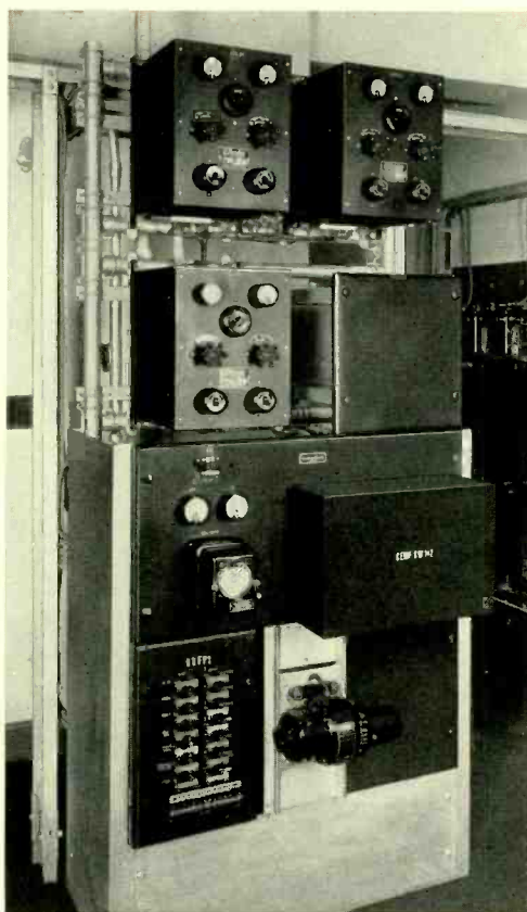
Fig. 4—An automatic power plant is included in the equipment for the 360-A unattended office
