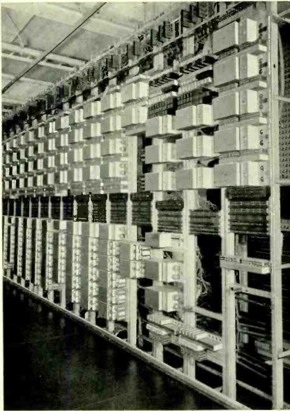
Fig. 8—A typical line of repeater bays
