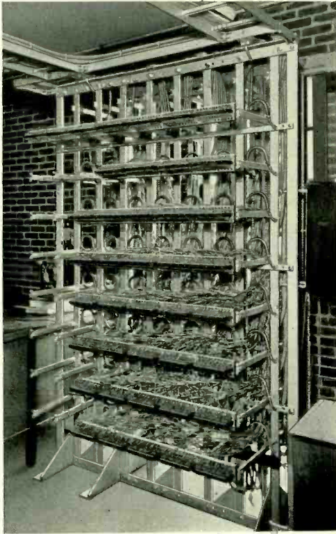
Fig. 2—Office side of combined distributing frame used with 360-A unattended offices for small communities
