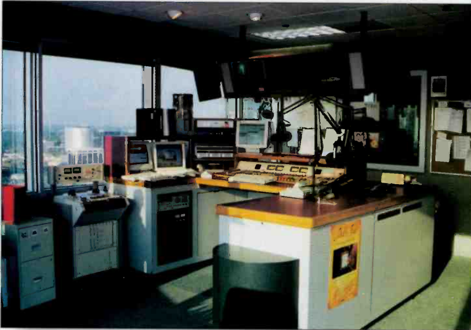
If studios are built with similar designs and consoles given similar layouts, operators working at more than one station will be more comfortable in different rooms. Photo by Richard Gerlovich.
