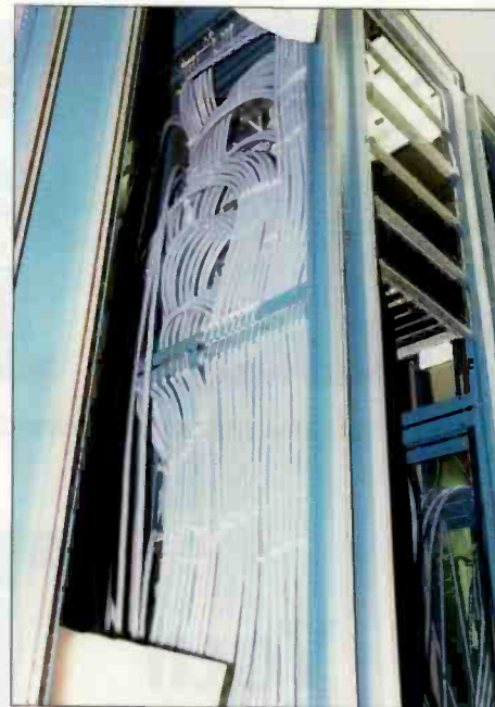
Multiple DAs result in a substantial amount of cabling, as shown in this installation. All the DA connections were connected to punch blocks through multipair cables. All of this was removed for the routing switcher installation. Photo by Robert Reymont.
