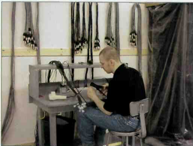
Assembling cable and preparing wiring plans off-site will facilitate the installation process.
