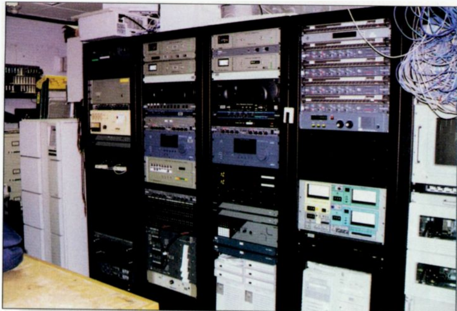
Central UPSs can be located in the rack room. In this installation, they are to the left of the racks. Photo by Richard Gerlovich.
