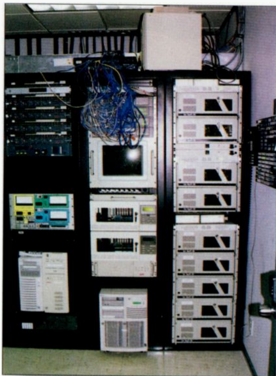
Installing all the computer audio servers in one room makes maintenance easier. It also removes a noise source from the studios. In this installation, the office LAN servers are at the bottom of the first rack. Photo by Richard Gerlovich.
