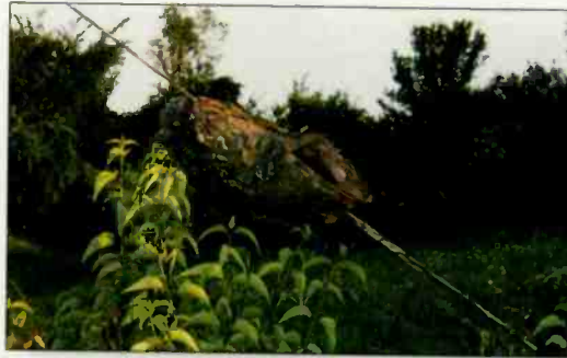
Keep vegetation around a tower under control. Before the tree in this photo was cut, the guy wire had been pushed several feet from its correct position.
