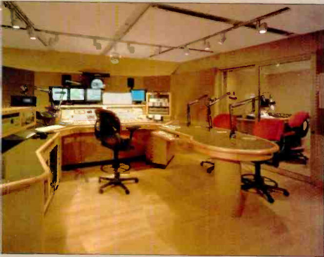
Each of the four on-air control rooms has an adjacent screenar/producer booth.
