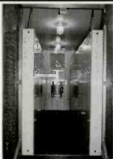
WCBS / WFAN 2 X 30KW AM DIPLEXER INSTALLED IN KINTRONICS PREFAB BUILDING
