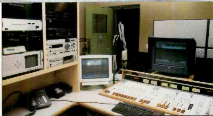
The main production room handles most of the station's production needs.
