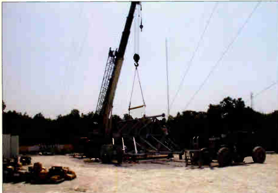
The chosen transmitter site should provide adequate coverage of the desired signal area, which may not necessarily be the city of license.
