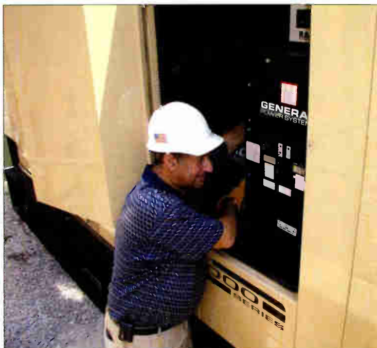
A backup power generator is an essential item at a transmitter site, particularly in remote locations.
