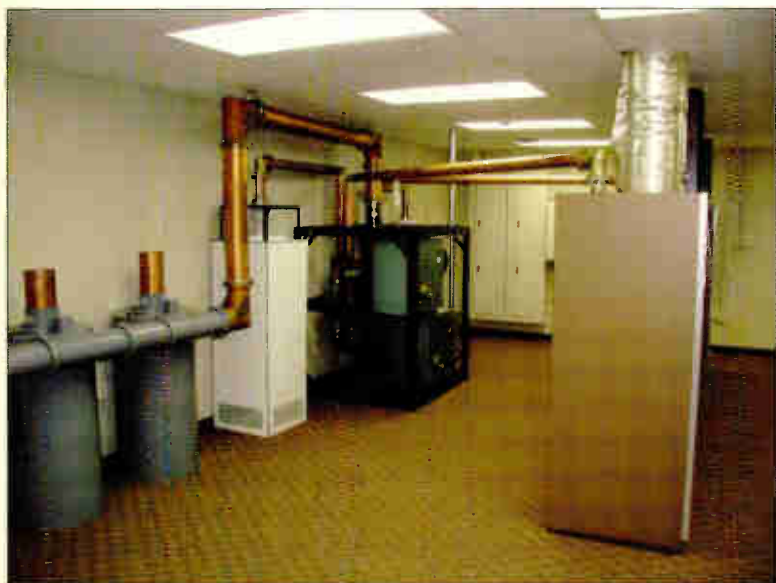
A clean and organized transmitter site makes a more efficient work environment, particularly during emergency maintenance.
