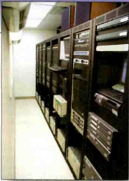
The rack room houses nine equipment racks, plus two open-frame racks for the office networks and phone system.
