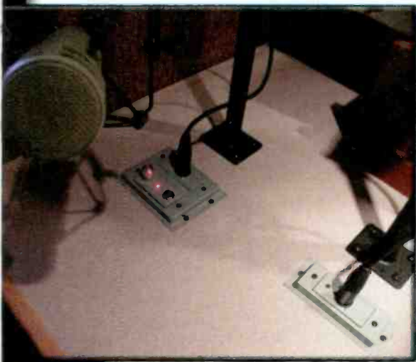
Studio Hub jack panels are placed at each mic position for a headphone jack and control.
