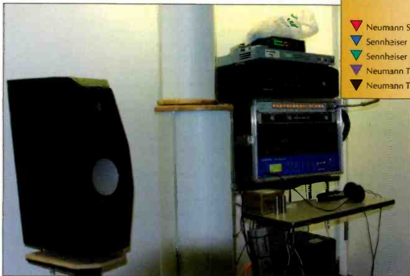
The transmission rack housed the Harris Neustar encoder, APT codec, Sony DAT and some stereo confidence monitoring equipment.
