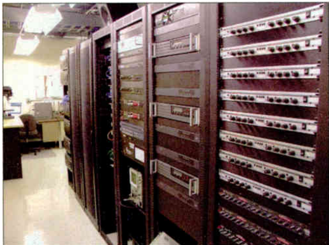
Because the studios are mostly self-contained, the rack room houses a minimum of equipment.
