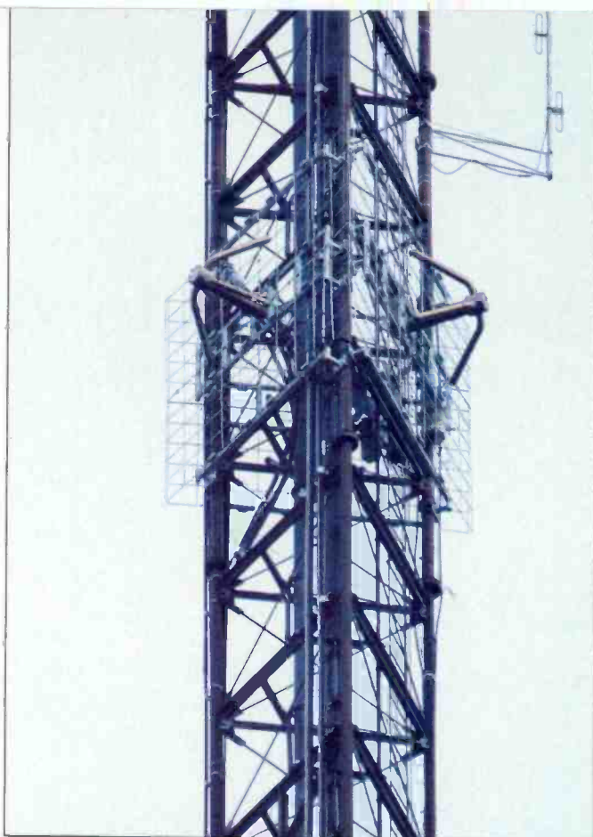
The ERI panel antenna for WDPR sits at the 880' level on WPTD's tower.
