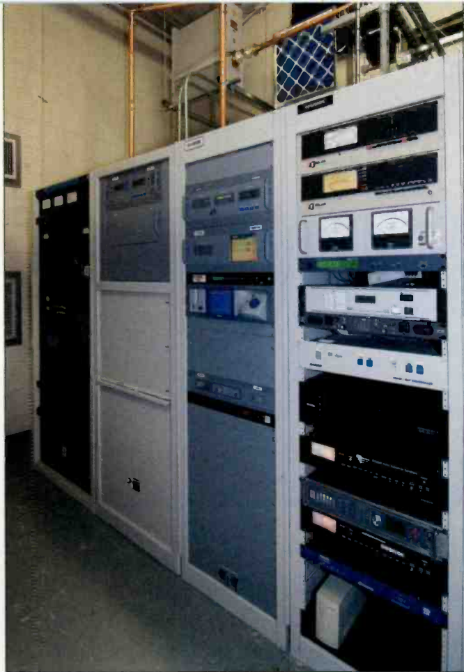
The WDPR transmitter (original pre-Flexstar configuration).
