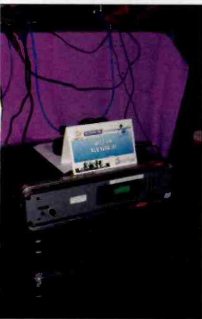
The ISDN codecs are placed between the stations using them.
