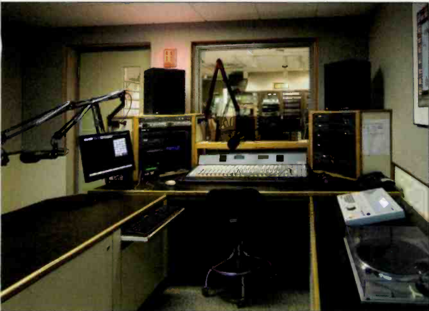
This is the production studio with a PR&E console, Enco DAW and Vistamax routing switcher. Only a portion of the extensive CD library is visible.
