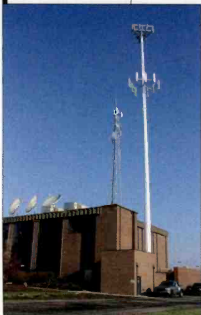
If a tower already exists in a suitable spot, wireless carriers are usually eager to lease space.
