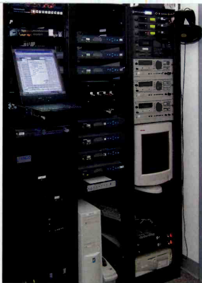
The Enco DAD automation system, satellite downlink receivers and webcasting.
