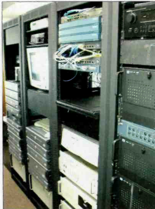
The Frederick facility also serves as the Nassau IT hub for this station and the Reading, PA, station.
