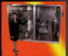
High-Power Antenna Tuning Units
