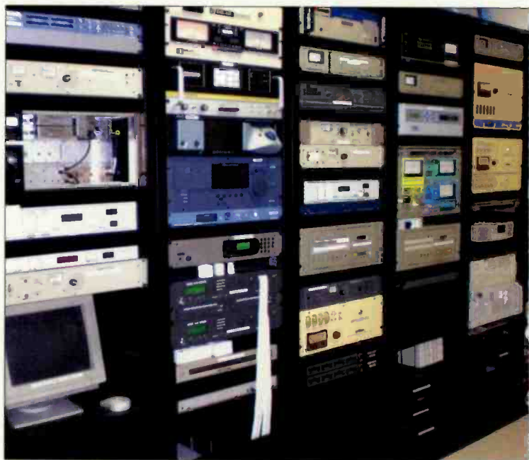
A rack row in the technical operation center houses the on-air processors, RF monitoring equipment and EAS encoders/decoders.
