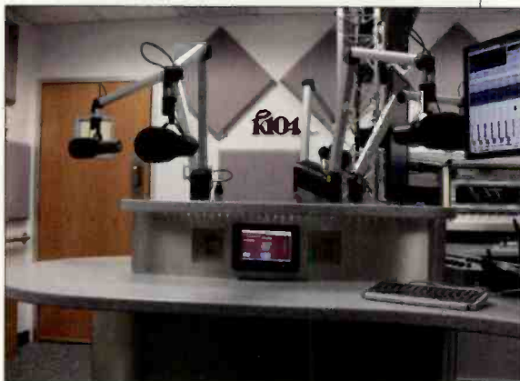
The mic cluster installed at KKDA.
