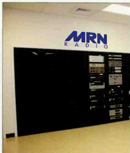
The technical operations center, in the engineering shop, is adjacent to the climate-controlled work bays where the remote trucks are housed. One truck can be seen through the window.
