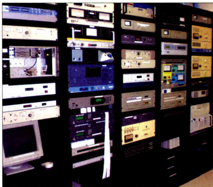
A rack row in the technical operation center houses the on-air processors, RF monitoring equipment and EAS encoders/decoders.
