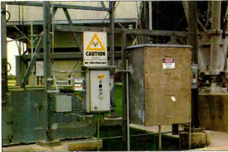
The unit installed at one of Richland's sites.
