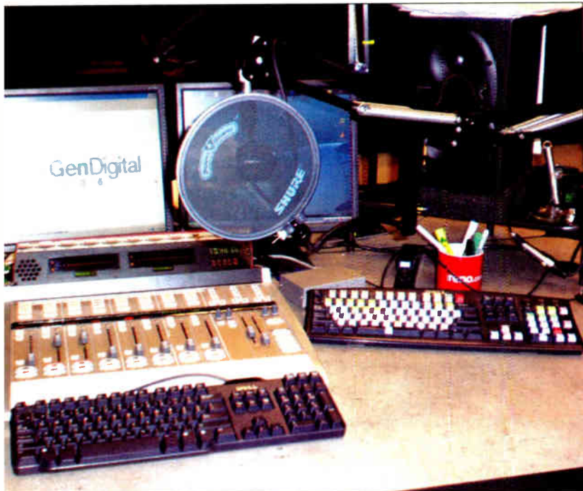
The set-up in Production 1 shows the typical console and automation system layout in each studio.
