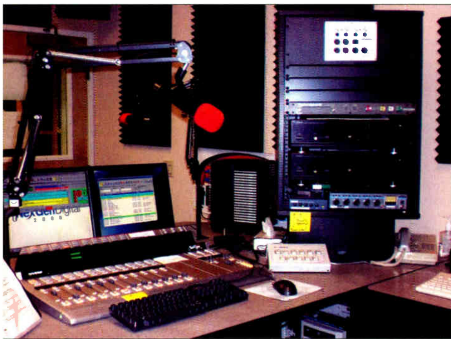
The KODS-FM studio is centered around a Harris Netwave console and Prophet Nexgen automation. Rack equipment at KODS includes Denon CD players and a Gentner Digital Hybrid II phone system. A Harris World Feed panel for plug-in systems is integrated into the top of this rack.
