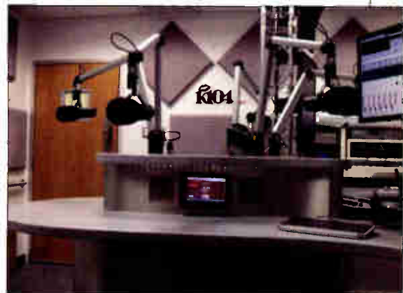
The mic cluster installed at KKDA.
