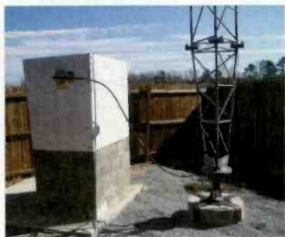
High-Power Antenna Tuning Units
