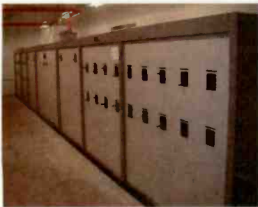
CUSTOM PHASOR INSTALLATION
