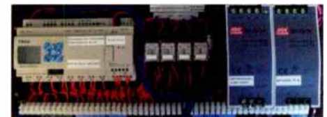
Figure 2: PLC-Based Antenna Controller
