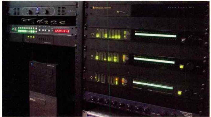
Kramer video matrix switcher (left) for managing studio LCD monitors and Wheatstone Blades (right) for audio and logic routing
