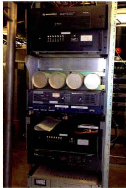
Figure 4. 2-way, RPU receiver, and ICR transmitters located at Pleasants Peak
