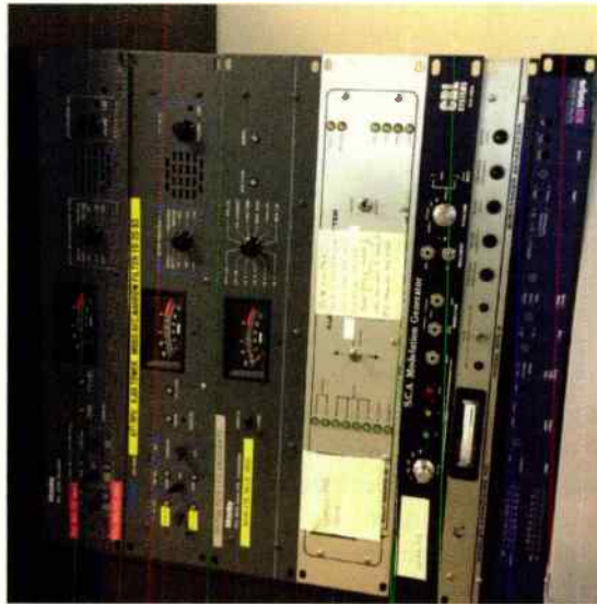
Store rack-mounted gear on its side for quick removal.
