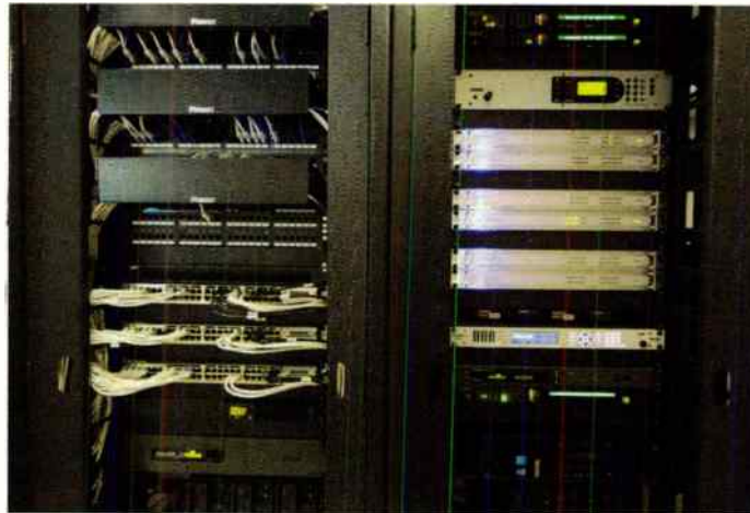
Server Room 407 has two racks dedicated to radio. Middle Atlantic DRK series racks had cable management in the front and back, giving it that finished look.
