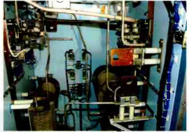
When inspecting the inside of a phasor, the transmitter power should be turned off.
