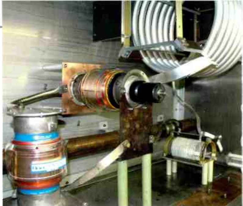
The inside of an ATU or phasor should be clean.
