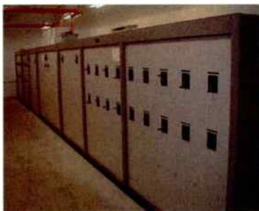
CUSTOM PHASOR INSTALLATION
