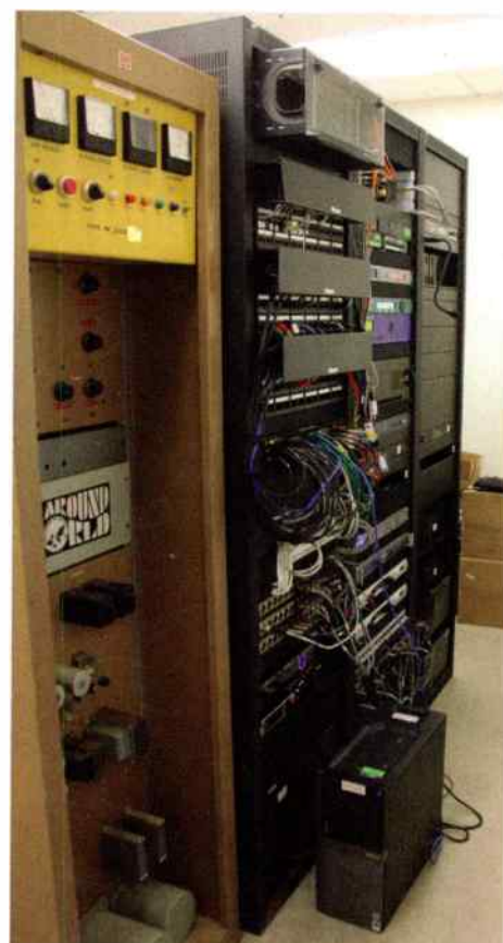
The rack room, seen with an old transmitter that will be used as a back-up.
