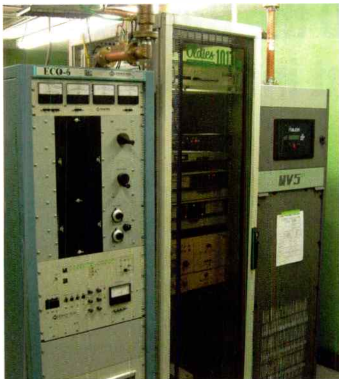
WIOE's NV5LT FM transmitter features a modular design for redundancy, on-air serviceability and high AC-to-RF efficiency.
