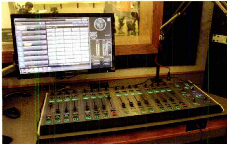
Lawo and WideOrbit in Air 2. Installation was simple — just a few cables.
