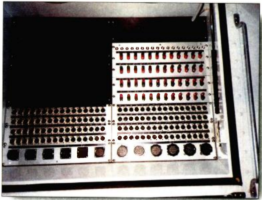
The majority of internal connections are available through patch panels for convenience and maximum flexibility.
