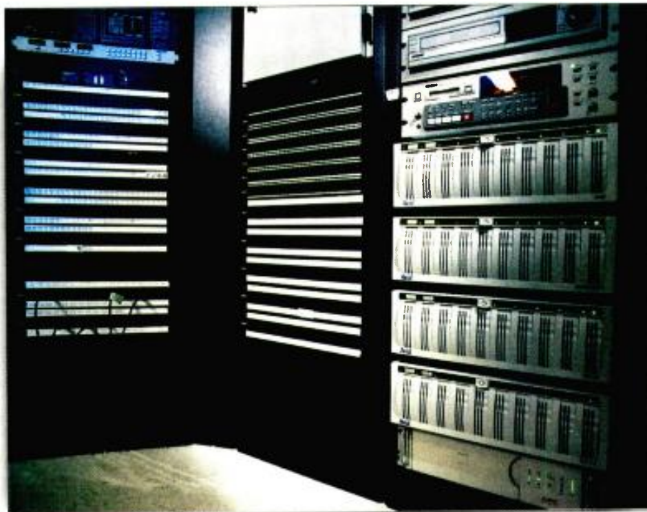
180Gb of shared fiber channel storage in the central machine room. Photo courtesy of Odyssey Network.
