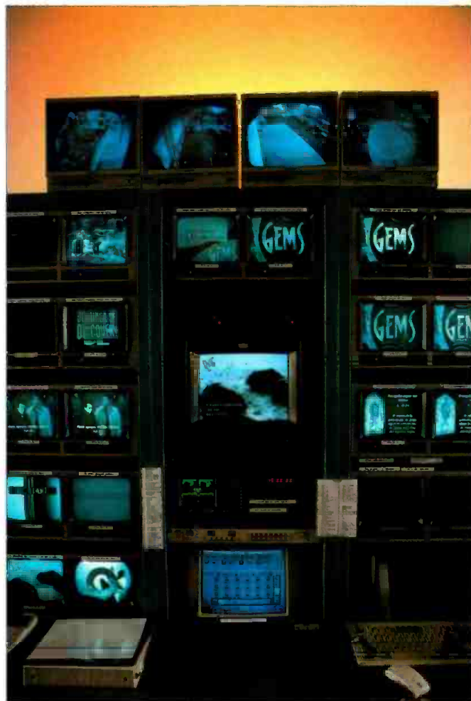
Computer monitors, test equipment, systems status and video signals all need to be networked in today's master control environment. Photo courtesy Globecast.
