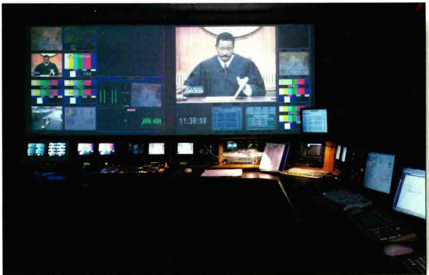
The design team incorporated a 16' x 7' projection screen (shown above) into master control, displaying output from two Miranda Kaleido multi-image processors. Images from up to 32 separate sources at one time can be shown on the wall.
