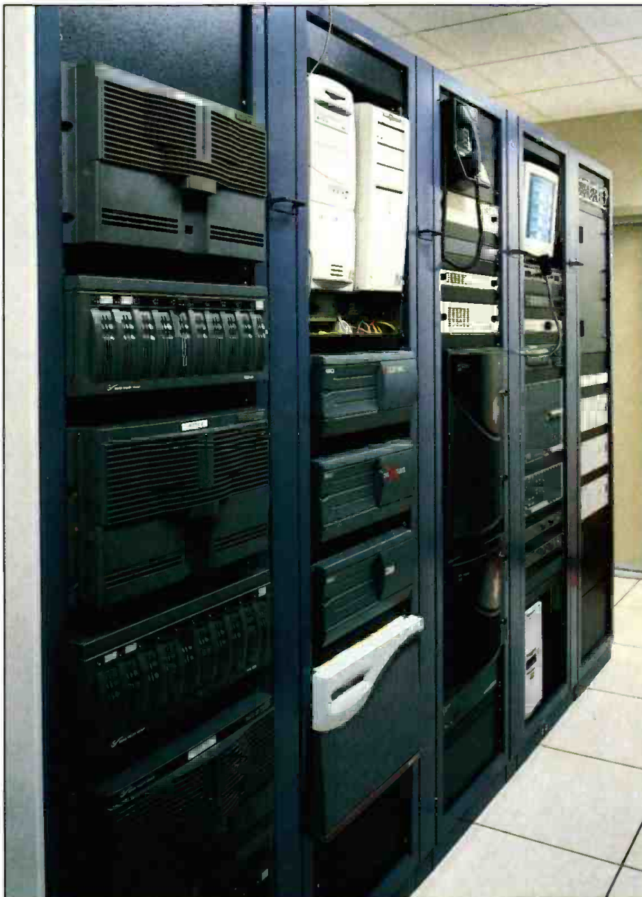
Shown above is a set of racks in KPDX's main technical core, containing the Profile XP server system, the Pinnacle and Quantel graphics mainframes, the main router, intercom and digital camera base stations.
