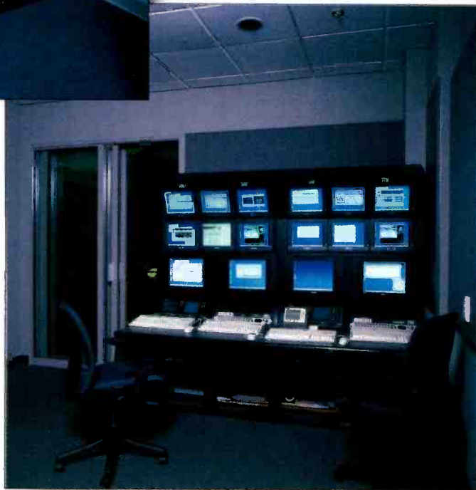
Below: The master control quality assurance station is used for encoding to all delivery systems, including fiber, terrestrial and the Internet, as well as sending material outside the facility.
