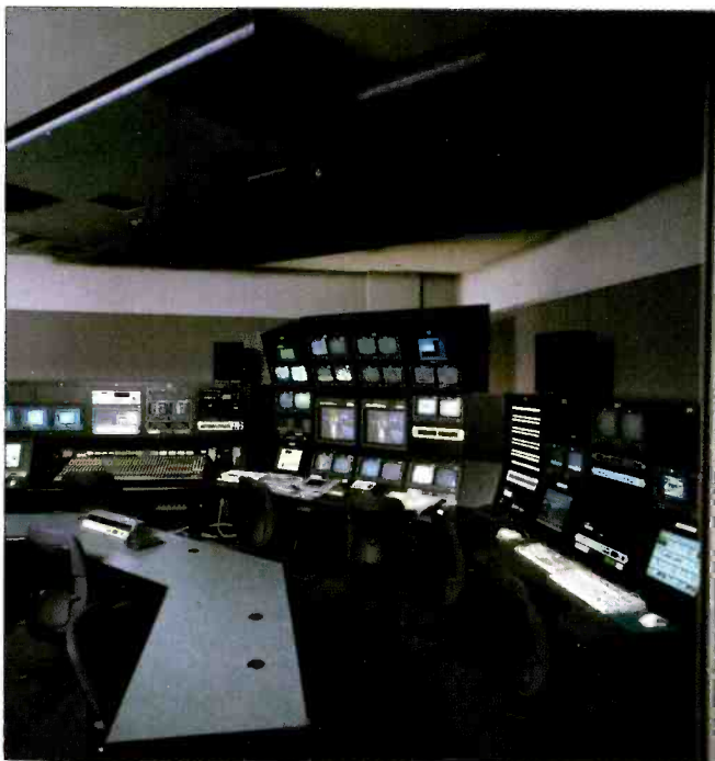
Control A, the largest of the four control rooms, features a Sony DVS7150 production switcher, several Pinnacle Systems' products and a Crest audio mixing board.
