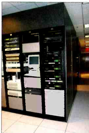
The righthand rack was customized by Microwave Radio Communications to provide WALA's STL/TSL with hot standby and space diversity features.
