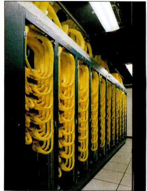
Router cooling and wiring must coexist.
