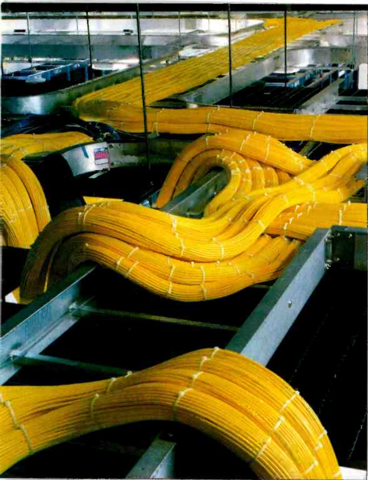
Large installations require careful attention to cabling plans.
