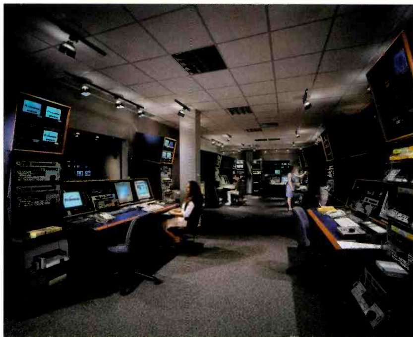
Pre-production areas are used for ingest of programming materials and the preparation of content for air. The pre-production area above is used to create individualized channel content, such as sports programming for FOX SportsNet.
