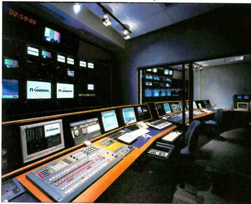
RNC created flexible "clusters" of multichannel control rooms to allow switching between individualized live programming and control of up to four channels in multichannel mode. The single-tier control room above includes a GVG M2100 master control switcher, GVG Profile XP servers, and Sony monitors and VTRs.
