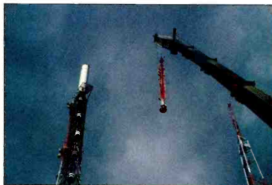
A crane lifts a superturnstile antenna for installation atop a DTV-panel antenna at KUAT-TV in Tucson, AZ. The three levels of batwing-shaped radiators identify the antenna as a three-bay superturnstile.
