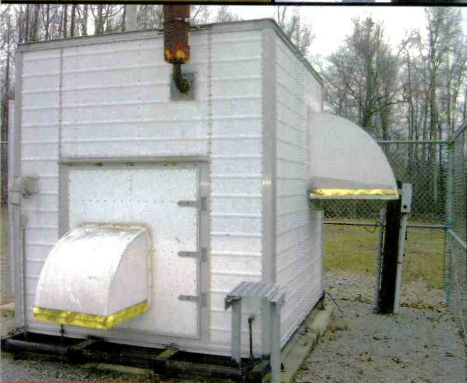
Left: Genset housing showing intake air louver in front and the exhaust on the right. Note the ice shield protecting the propane piping at the lower right side of the structure.
