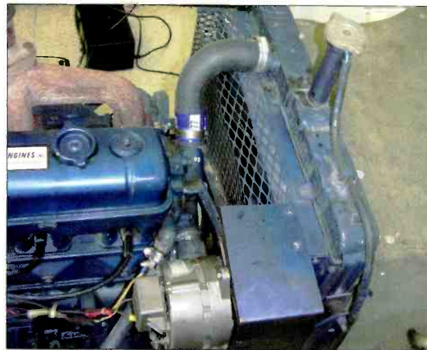
Check glycol level and the integrity of the hoses.
