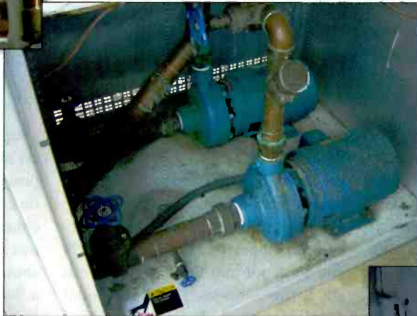
Pumps can be used alternately on a monthly basis. Valves and connections should be inspected for leaks.
