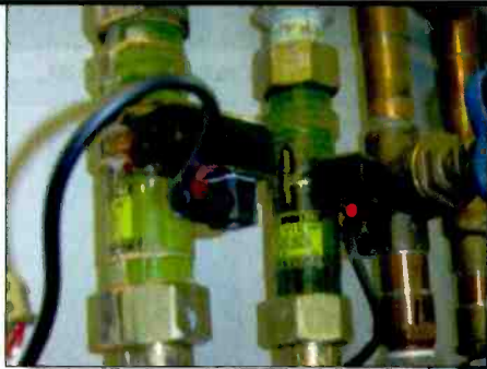
Flow regulators maintain the correct coolant flow into the IOT. The red LEDs indicate that the flow is above the minimum allowed.
