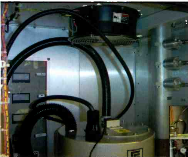
The power amplifier cabinet fan cools the top of the IOT's input cavity.
