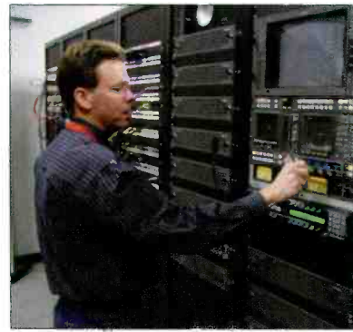
Although Rodeo Houston signal routing and machine control is fully automated, James Davidson, HLSR managing director of broadcast and audiovisual services, likes having the ability to monitor status with the flip of a switch. Photo courtesy Phil Kurz.
