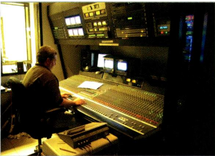
HLSR uses three separate audio studios to support its Rodeo Houston production; in the main room is a 64-input Amek Recall console used to control all live feeds, and Yamaha DM2000 consoles are the centerpieces of the surround and concert audio rooms.
