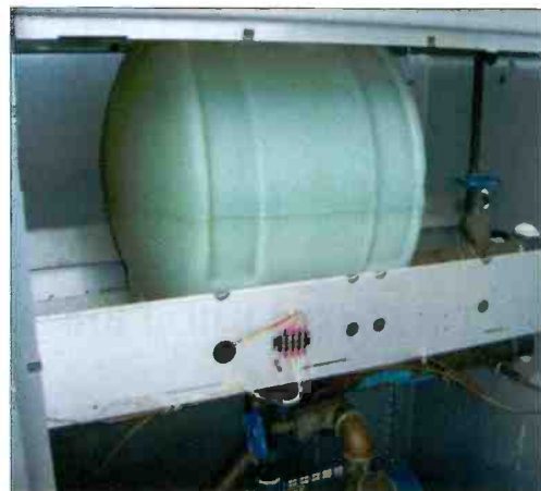
With the removal of the pump module's side panels, the coolant's reservoir tank is ready for visual inspection.
