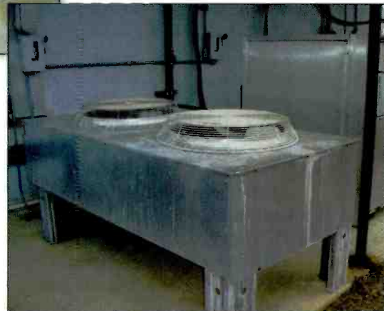
This photo shows the heat exchanger with the pump module at the back. Air is blown upwards by the fan, and the radiator is underneath the enclosure at the air intake. The AC power switch for the fans is at the upper left corner.
