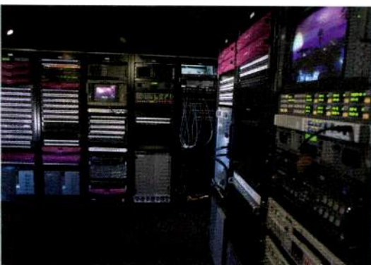
Trinity Broadcast Network's production and broadcast facility in Tustin, CA, features Stantron Broadcast E-Racks.
