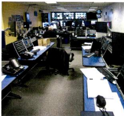
The main ingest area accommodates more than 125 feeds that come in daily and are converted in real time to a widescreen aspect ratio in both SD and HD by 10 operators.
