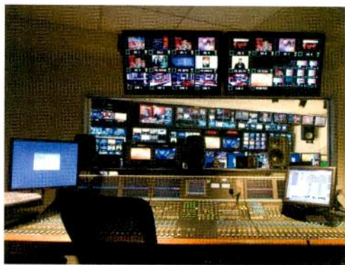
A fully networked Calrec Hydra audio spider system in the audio mixing room allows FOX to multiplex signals and combine a large amount of sources (wireless mics, audio recorders, etc.). The system also enables any of the facility's studios to access any audio console in the building.
