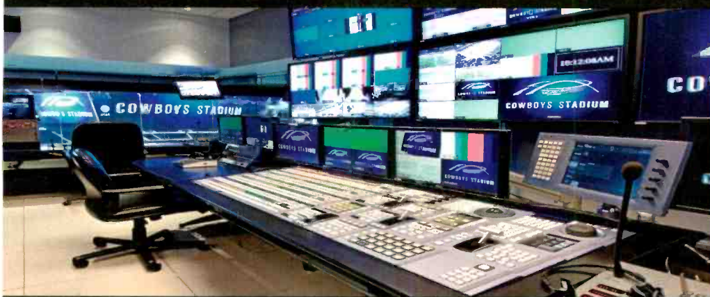
Dallas Cowboys Stadium Control Room features a Sony MVS HD Switcher
