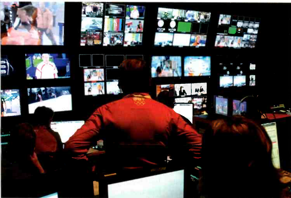
Six studios and seven control rooms were built in Vancouver at the IBC, including five main control rooms, like the one pictured here, to support the five main OBMC members' live coverage.
