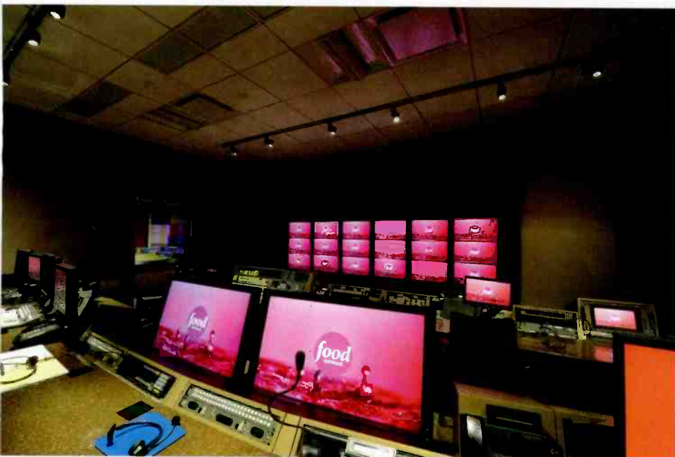
The refurbished HD control room features an innovative use of NEC LCD monitors at the front wall (six screens hung vertically) and two at the back row to allow producers a better view on what's happening in the studio during show tapings.
