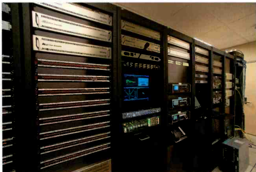
In the technical operations center, 12 card cages are loaded with HD (3G), SD, analog video, digital audio and analog audio distribution amplifiers.
