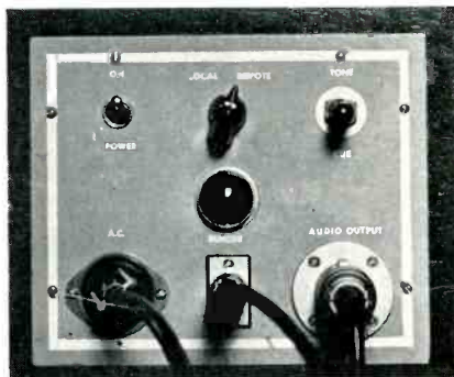
Fig. 2. Control panel of the signal device.
