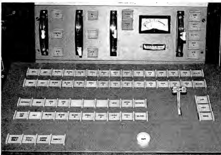
Fig. 1. Audio and video control panels for reed-relay master control switching.
