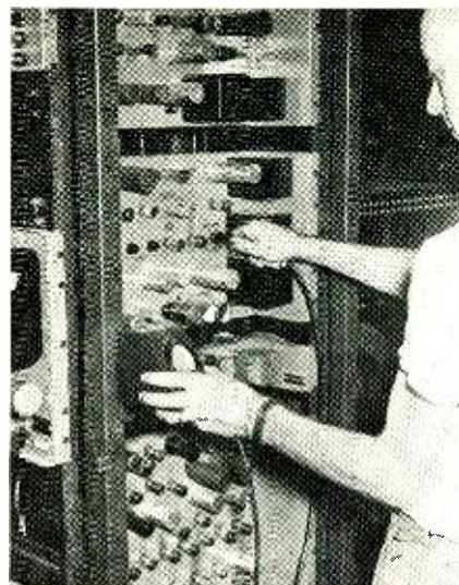
Fig. 7. Technician checks output voltages of power supplies mounted in rack.
